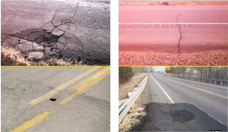
Common Culvert-Related Road Surface Distresses
