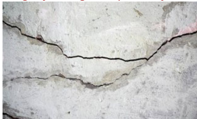
Severe cracking, wider than 1/4", with significant faulting
