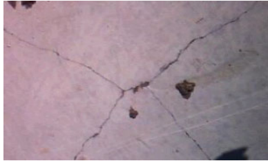
Mild cracking, no impact to flow
