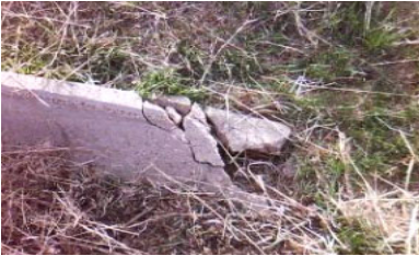
Mild damage to outlet
