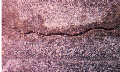
Moderate cracking, up to 1/4" wide, slight faulting or impact on flow
