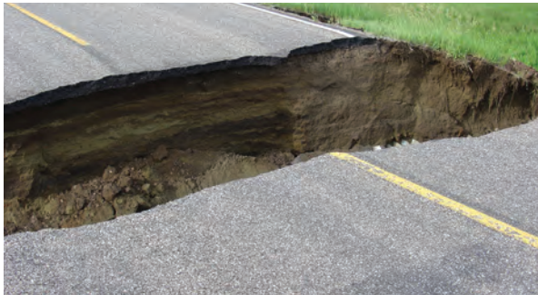
The collapse of a corrugated metal pipe culvert under state Highway 63 created this washout.
