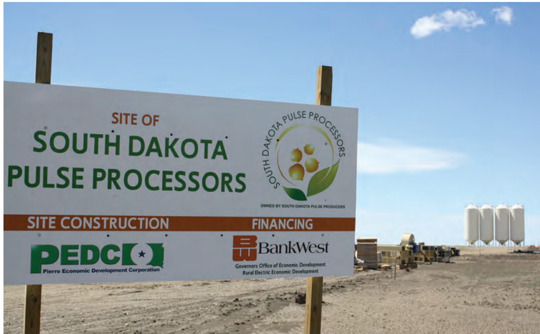
The South Dakota Pulse Processors plant in Harrold was under construction in May 2014.
