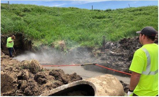
Chad Urban running the jetter and Dan Trost standing by the culvert end. Photos submitted by Steve Schneider, Highway Maintenance Supervisor for Flandreau/Madison 272 and William Burshiem, Lead Highway Maintenance Worker for Flandreau 277.
