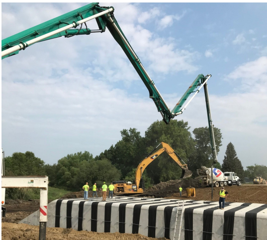
Mike Will and crew on top of 11ft. x 10 ft. pre cast box culverts on Highway 15 Project. Photo submitted by Mike Will, Watertown Area Project Engineer.
