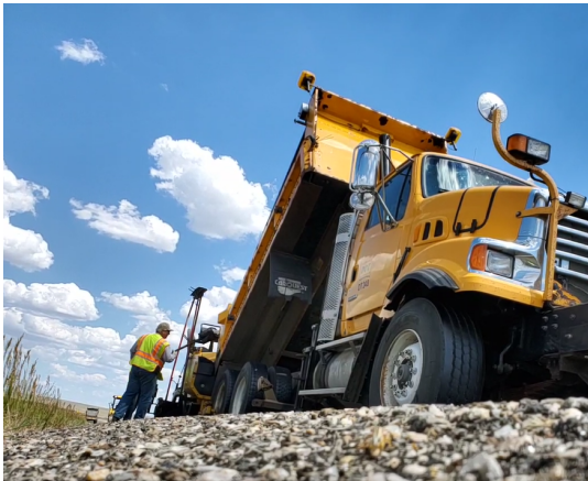
Larry Andersen, Lead Highway Maintenance Worker, working on Highway 34. Photo submitted by Luke Neville, Lead Highway Maintenance - Pierre Area.
