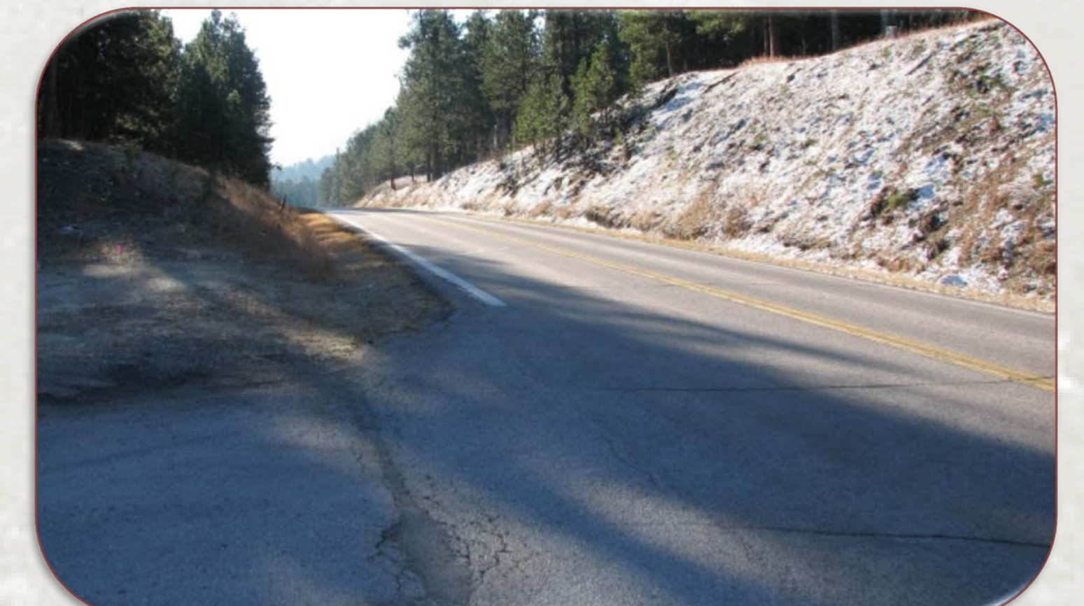
Limited Sight Distance Due to Slopes
