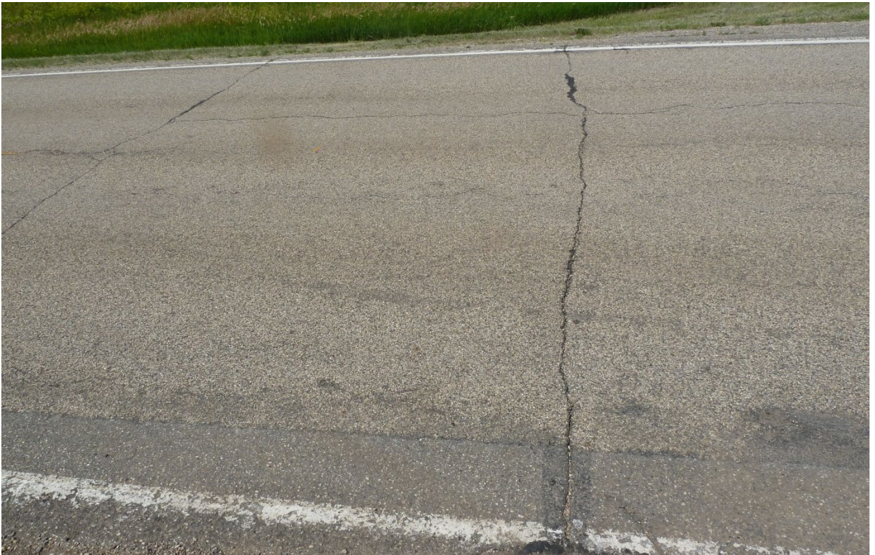
Figure 33: Medium Severity Transverse Cracking
