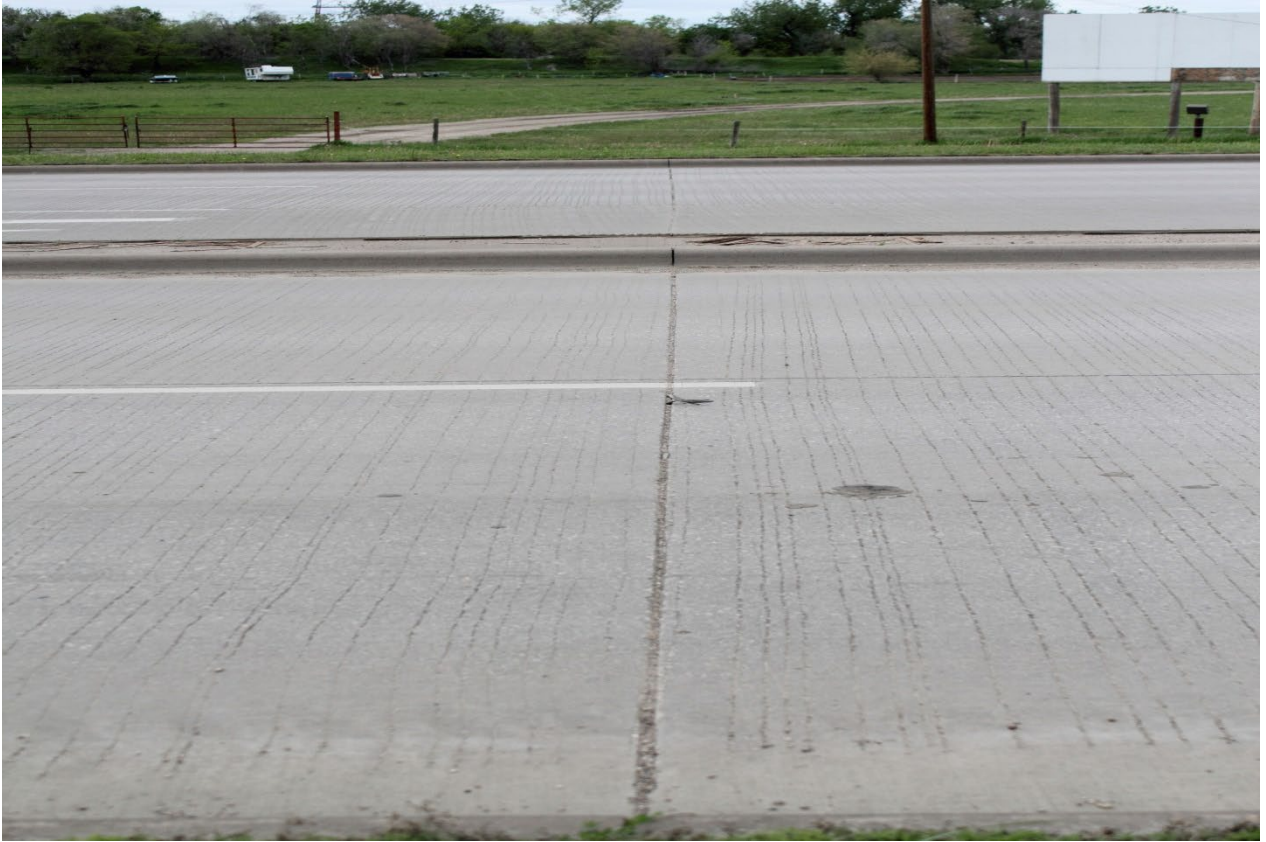
Figure 66: High Severity Joint Seal Damage
