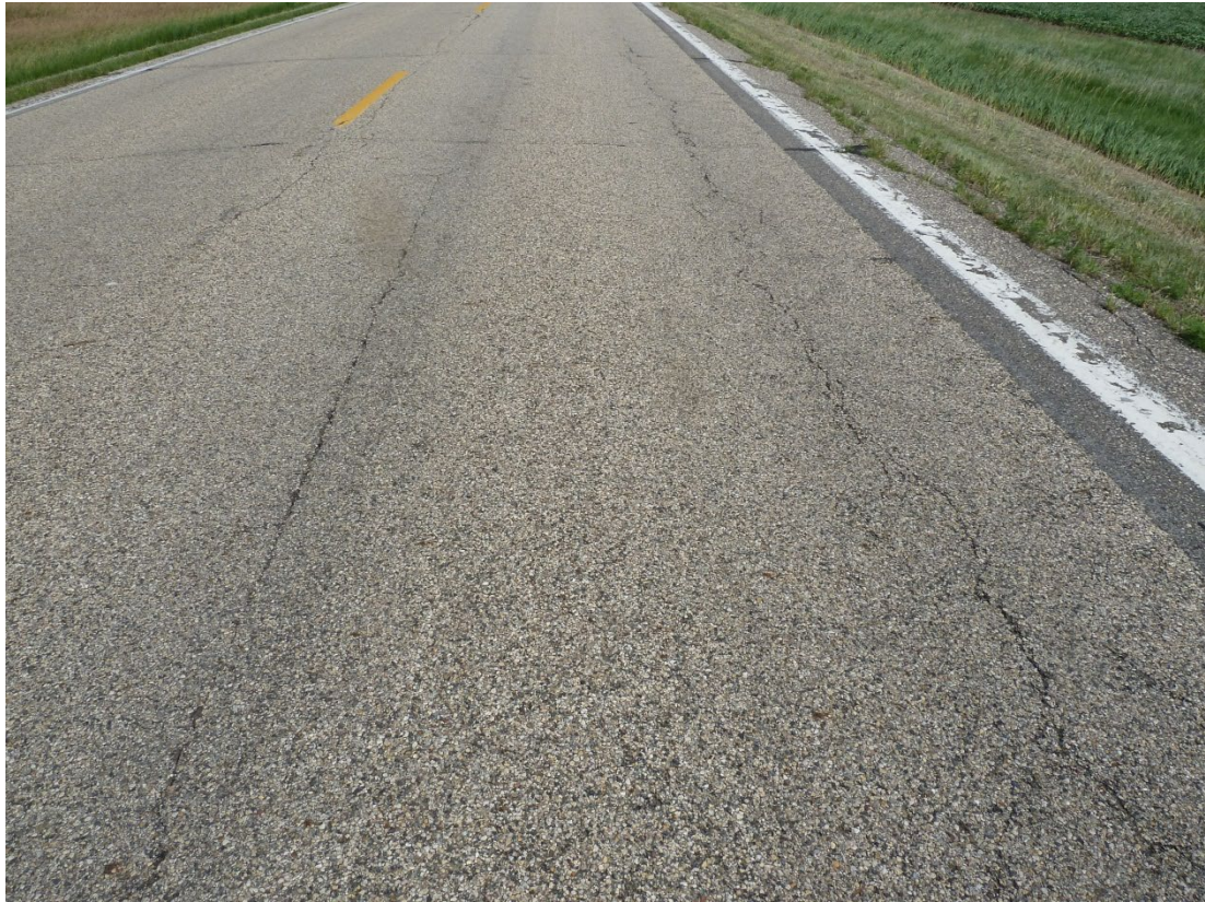
Figure 36: Low Severity Fatigue Cracking
