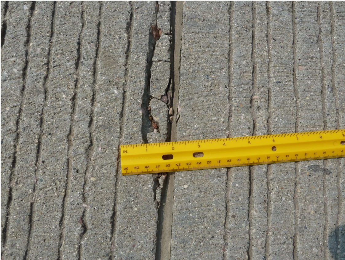
Figure 52: Low Severity Joint Spalling
