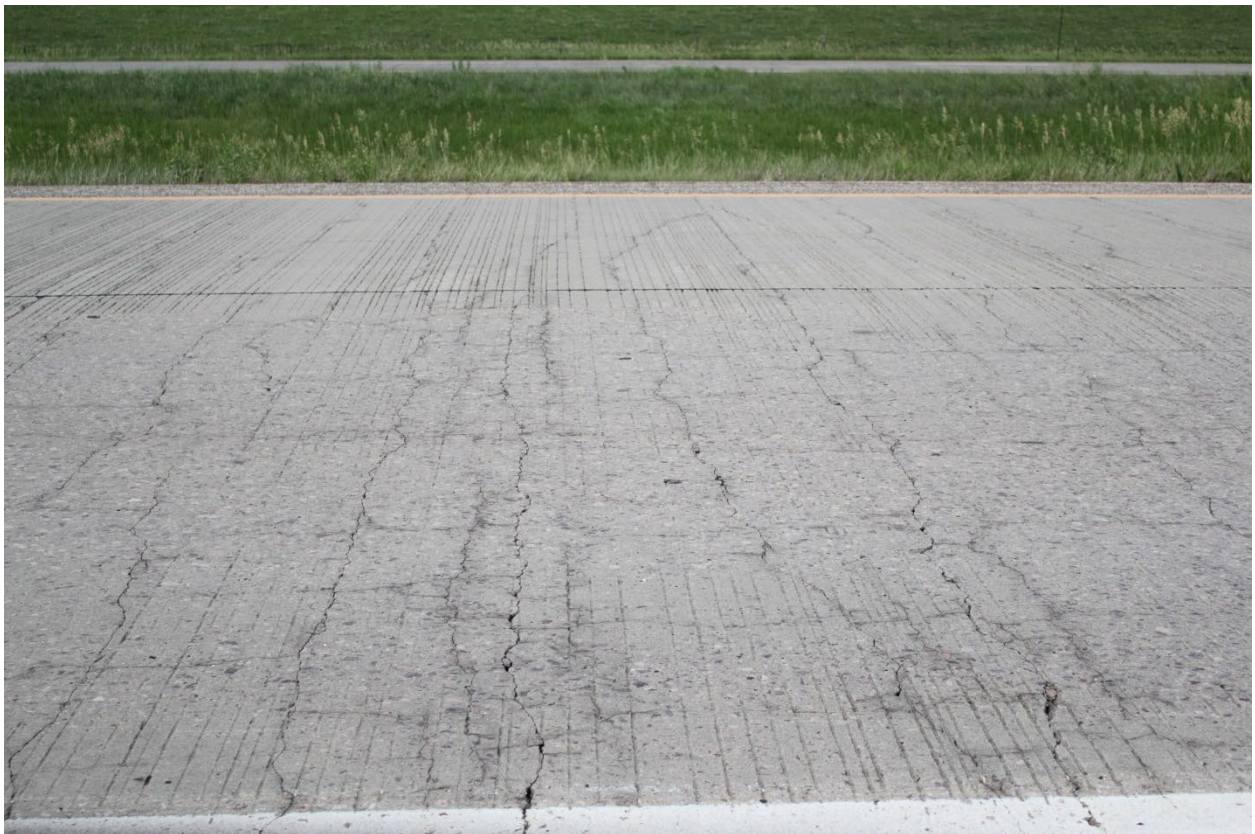
Figure 63: High Severity CRC Block Cracking
