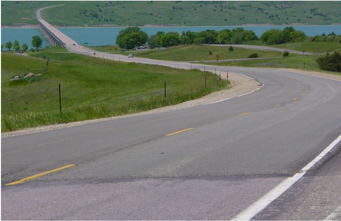
Figure 40: Low Severity Patching
