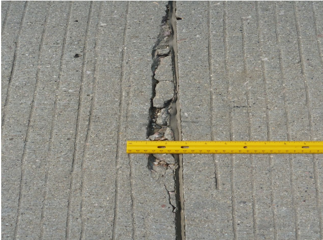
Figure 53: Medium Severity Joint Spalling
