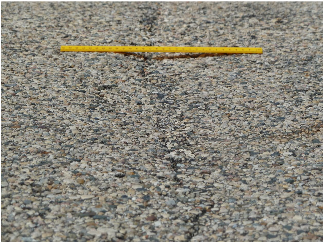
Figure 35: High Severity Transverse Cracking with Depression
