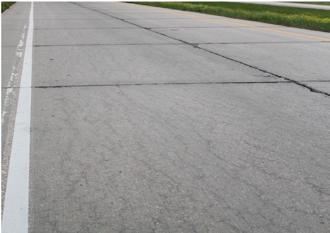
Figure 50: Medium Severity ASR
