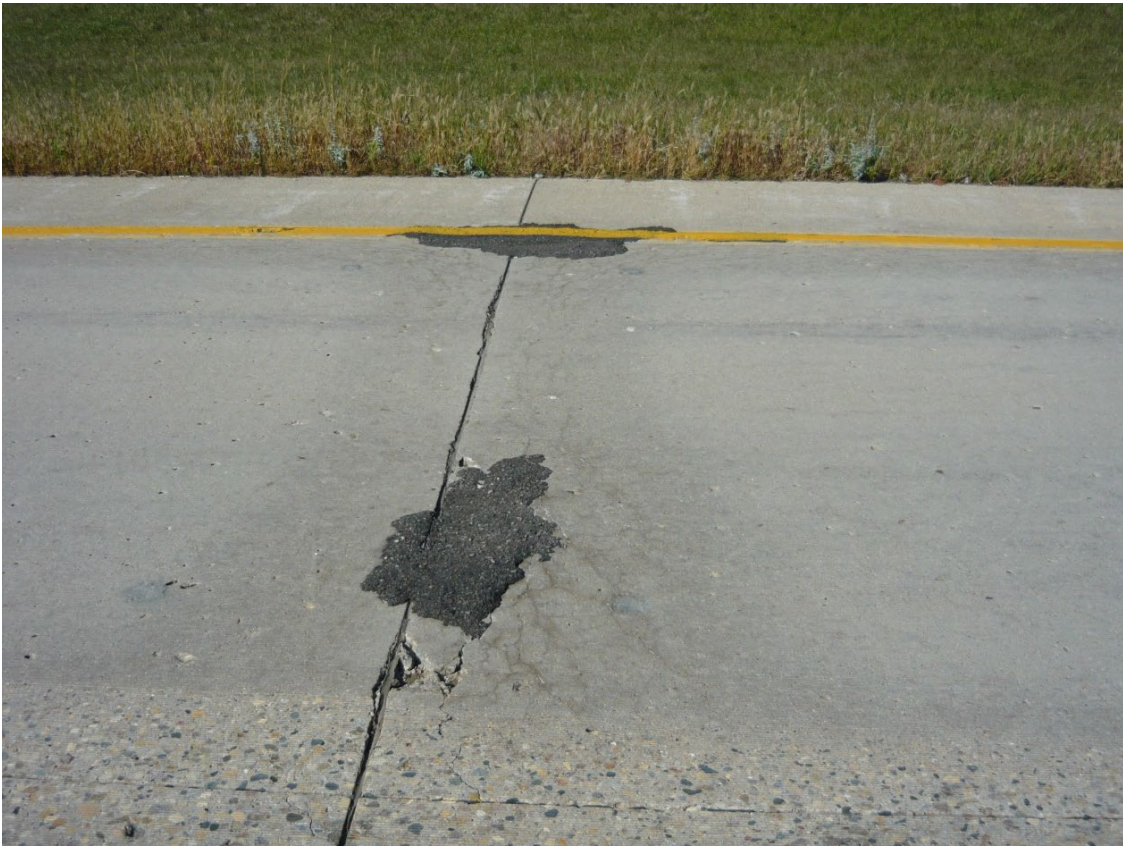
Figure 48: High Severity D-Cracking
