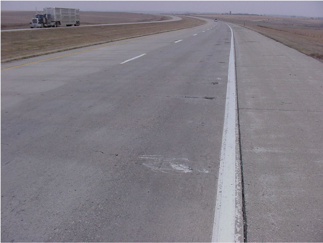
Figure 51: High Severity ASR
