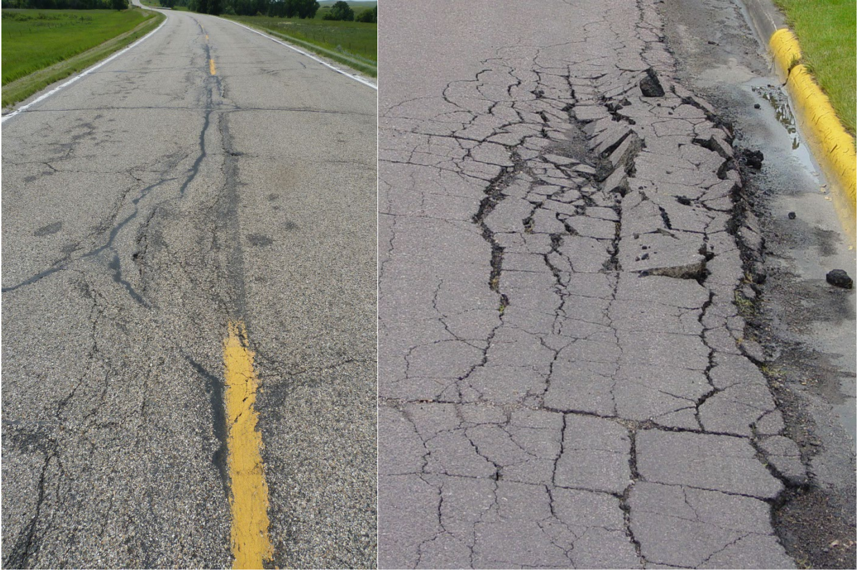
Figure 38: High Severity Fatigue Cracking
