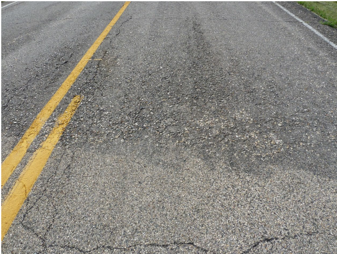
Figure 41: Medium Severity Patching
