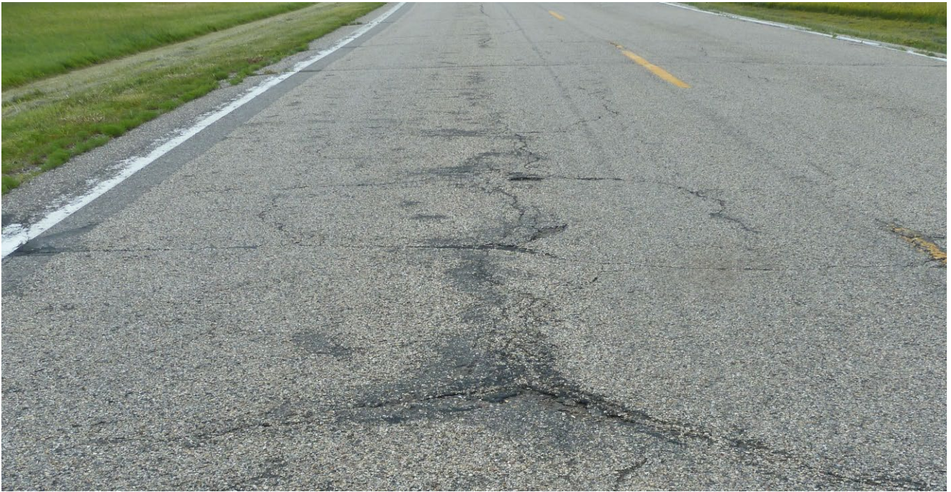
Figure 45: High Severity Block Cracking
