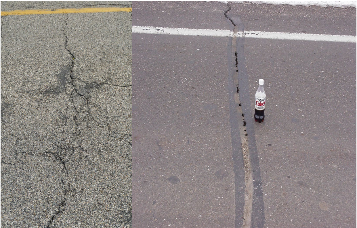
Figure 34: High Severity Transverse Cracking
