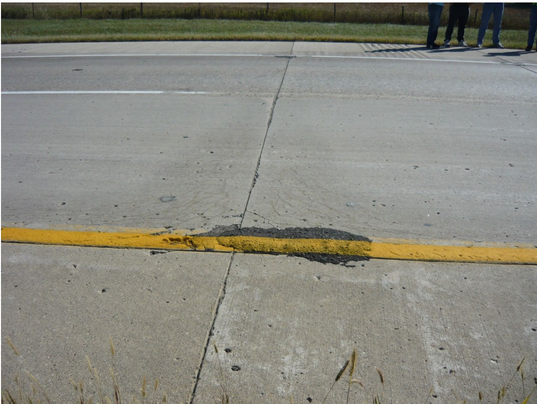
Figure 47: Medium Severity D-Cracking
