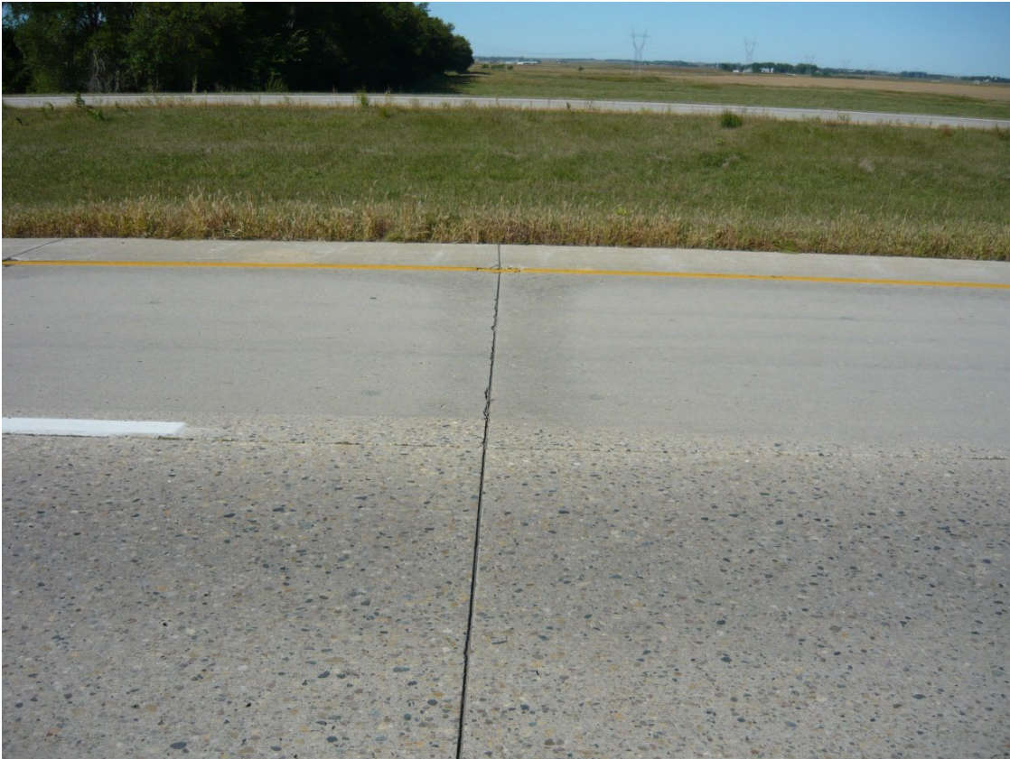
Figure 46: Low Severity D-Cracking
