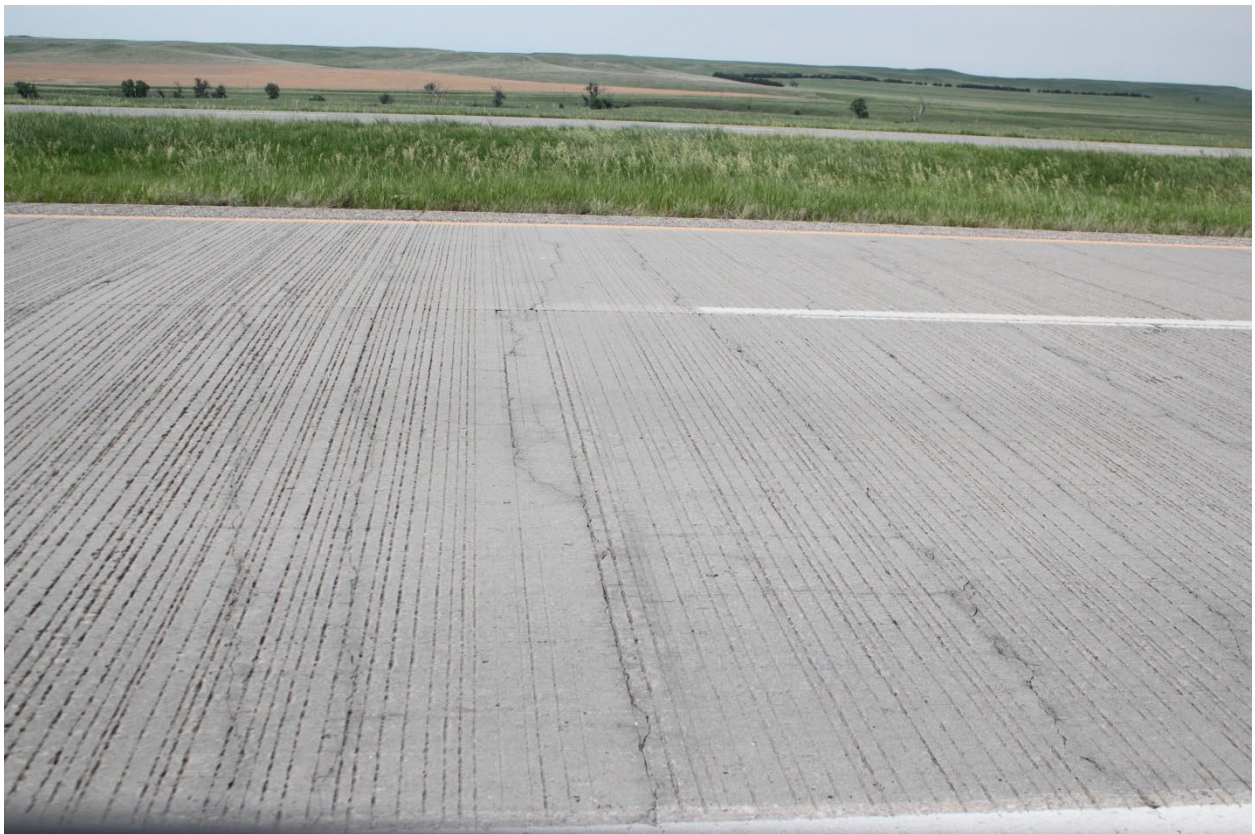
Figure 61: Low Severity CRC Block Cracking
