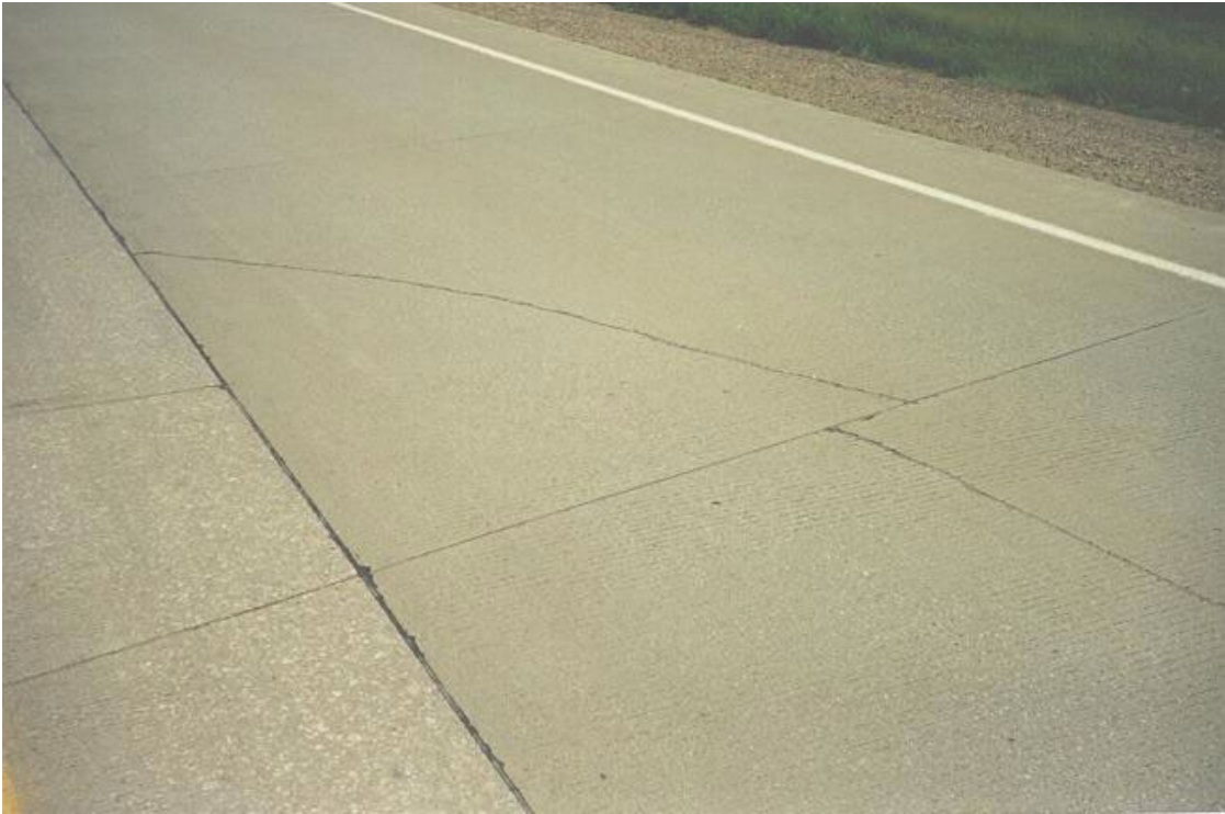
Figure 55: Low Severity Corner Cracking
