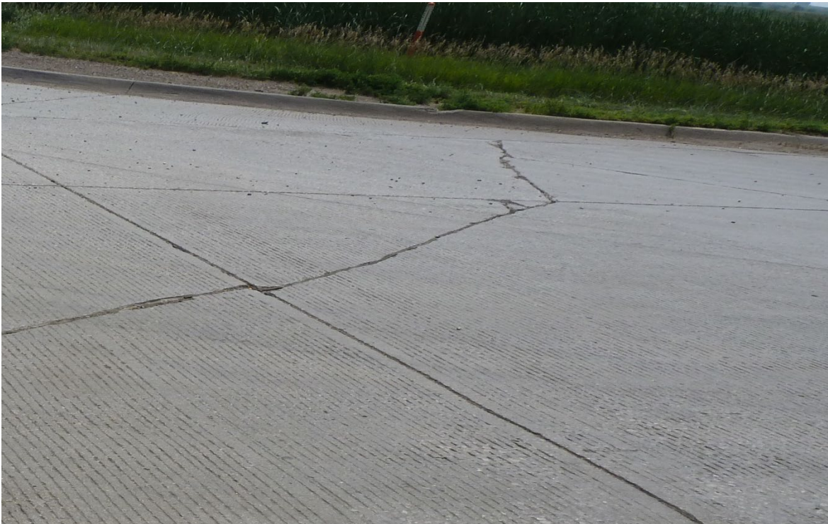
Figure 56: Medium Severity Corner Cracking
