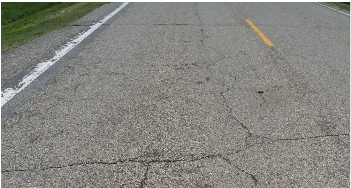
Figure 37: Medium Severity Fatigue Cracking
