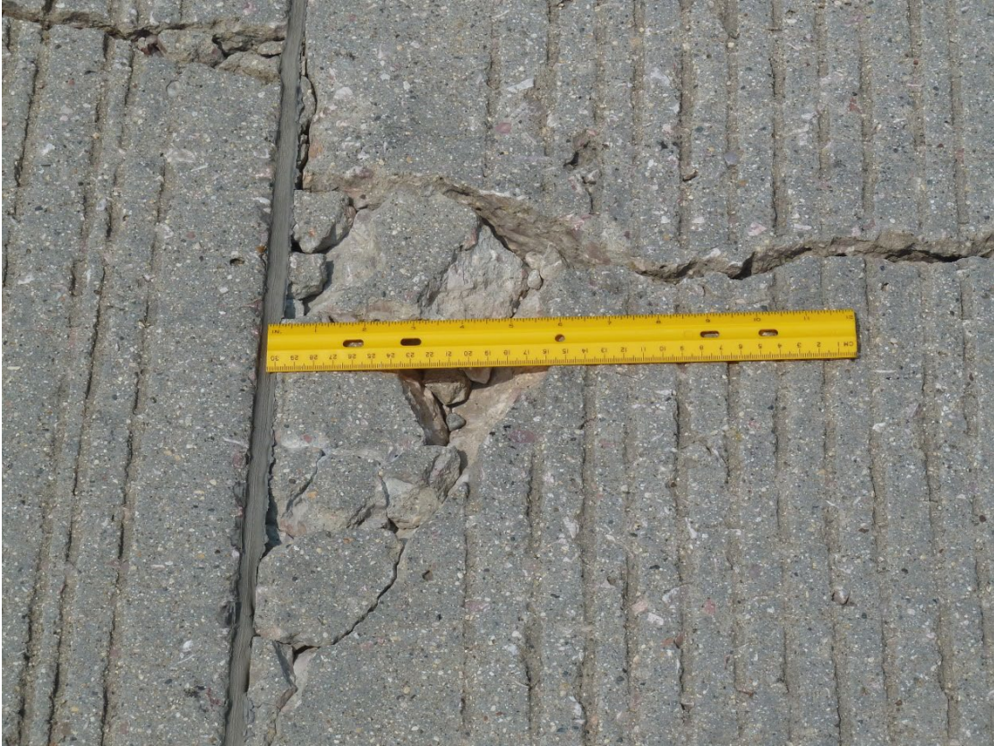
Figure 54: High Severity Joint Spalling
