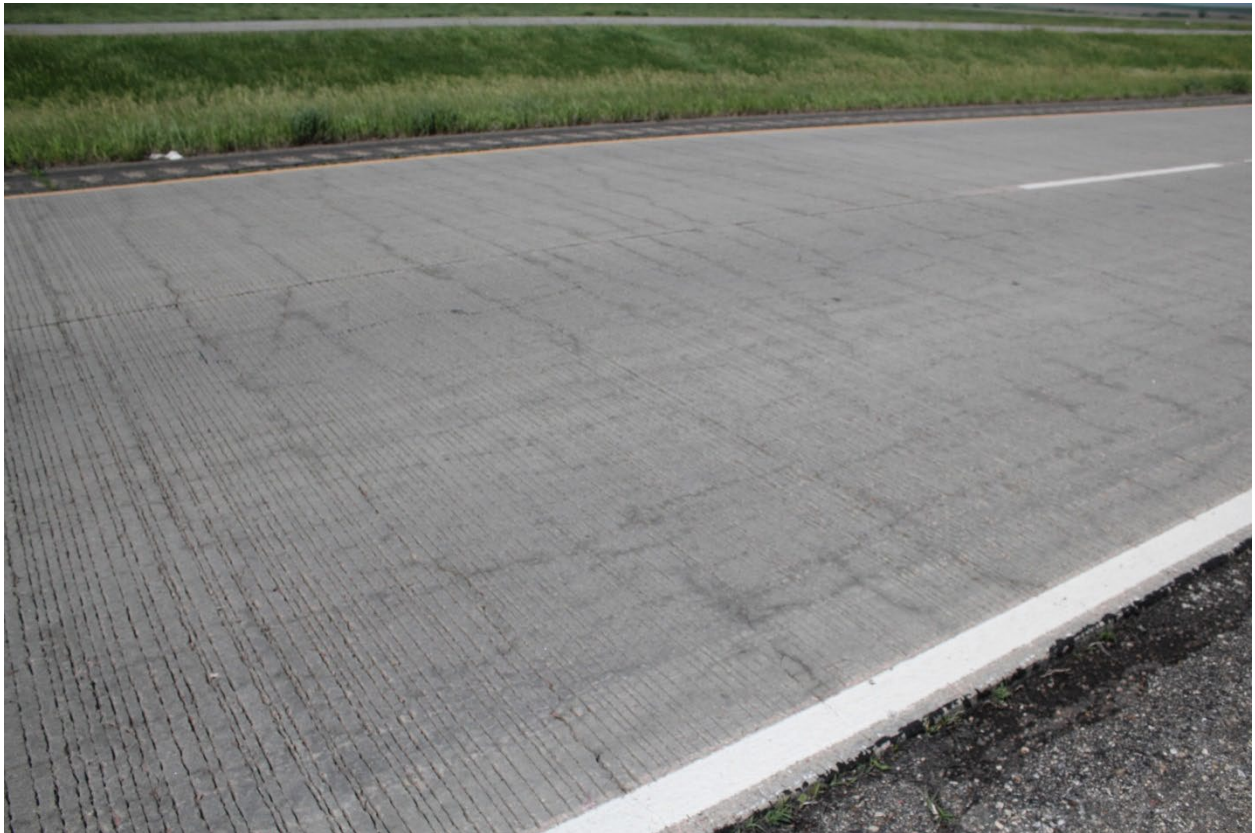
Figure 62: Medium Severity CRC Block Cracking
