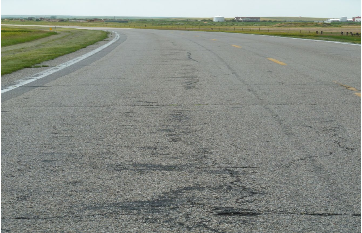
Figure 43: Low Severity Block Cracking
