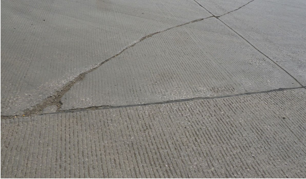
Figure 57: High Severity Corner Cracking
