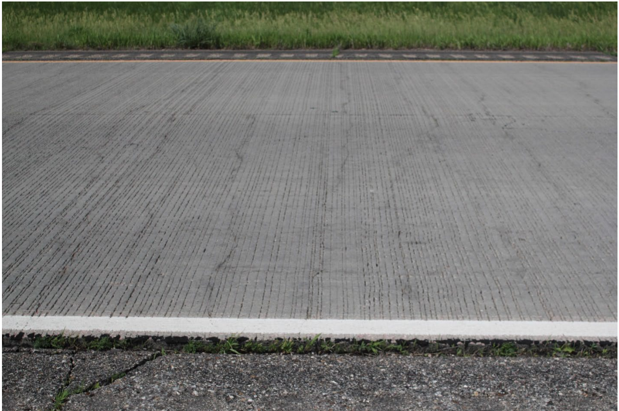
Figure 60: Low Severity CRC Block Cracking
