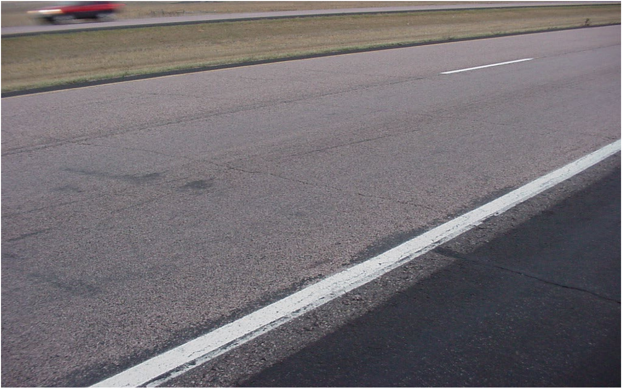
Figure 32: Low Severity Transverse Cracking
