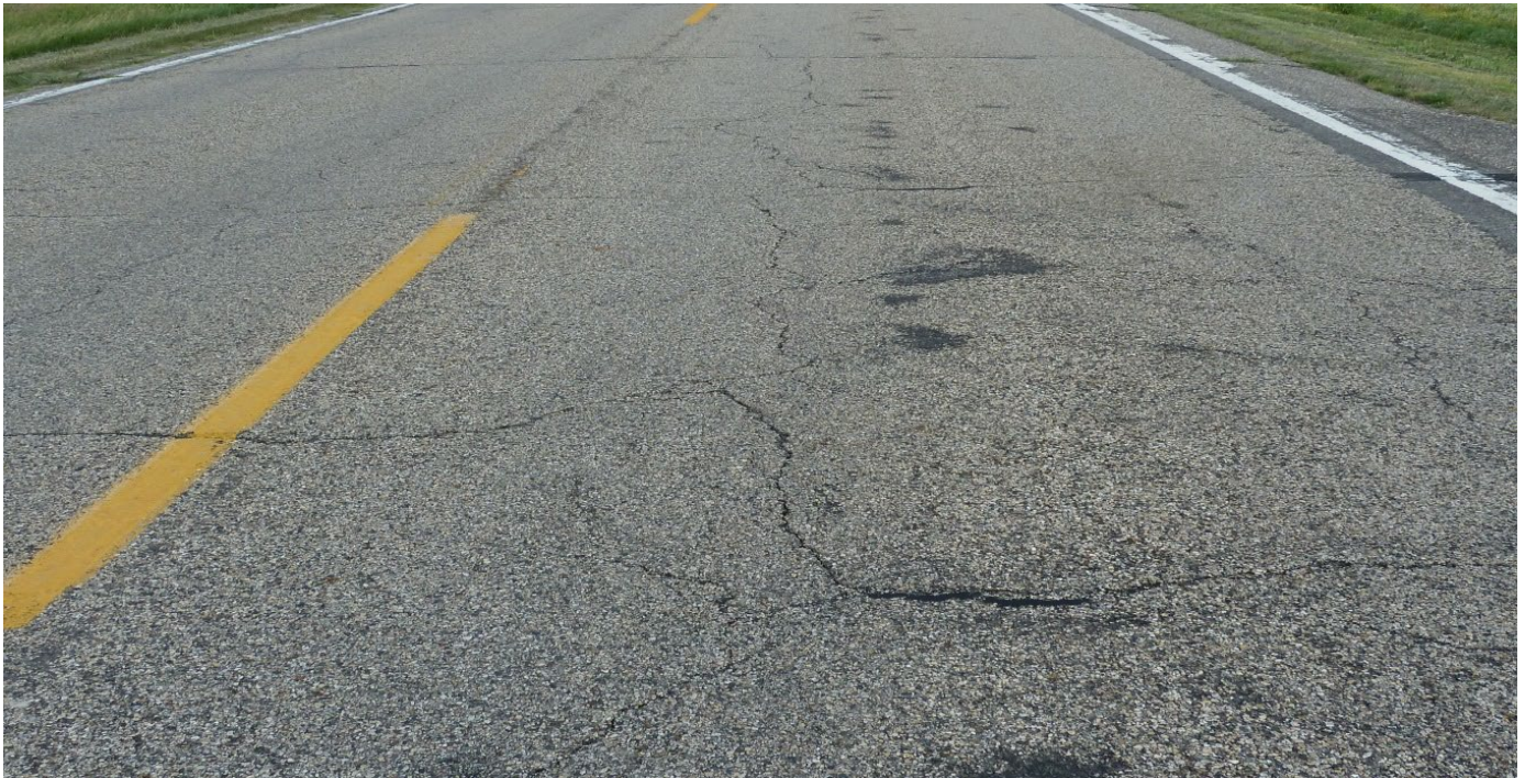
Figure 44: Medium Severity Block Cracking
