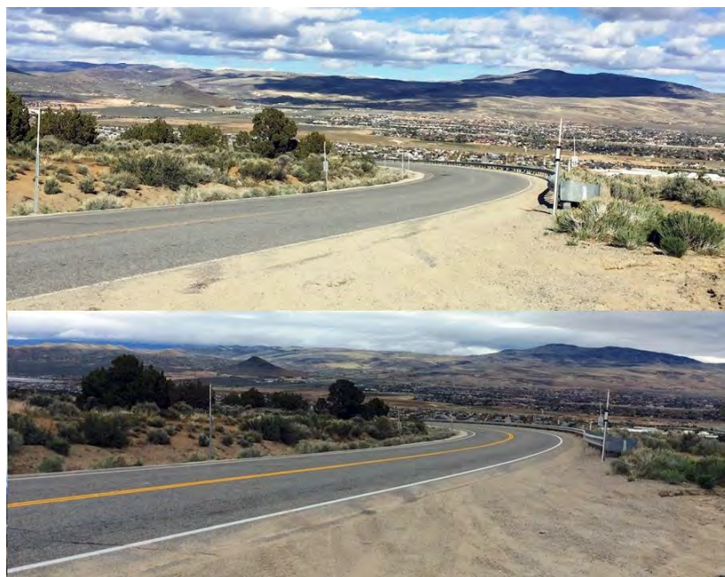
Figure 7. Before (top) and after (bottom) pavement marking maintenance by the Reno-Sparks Indian Colony Photo courtesy of Scott H. Carey, Reno-Sparks Indian Colony
