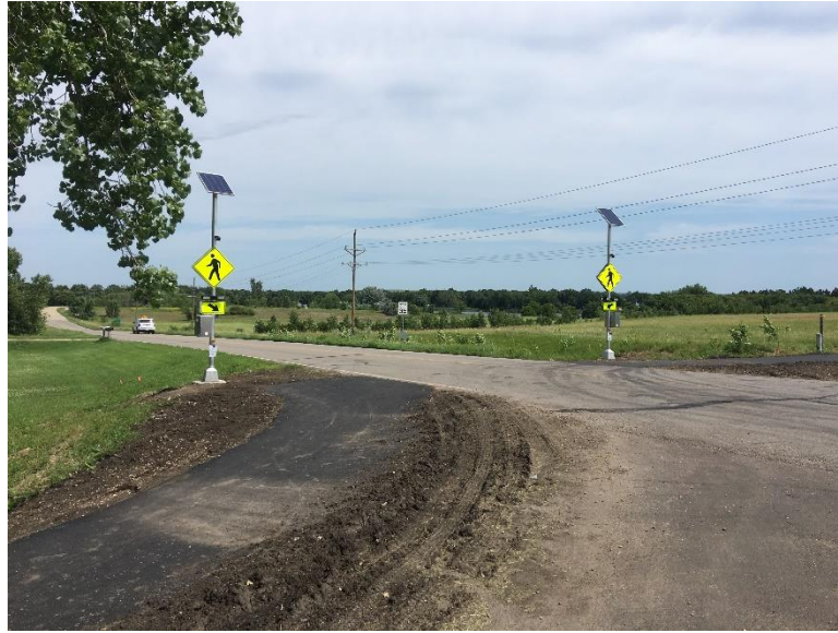
Figure 16: The project included the installation of a crosswalk with RRFB at the intersections.
