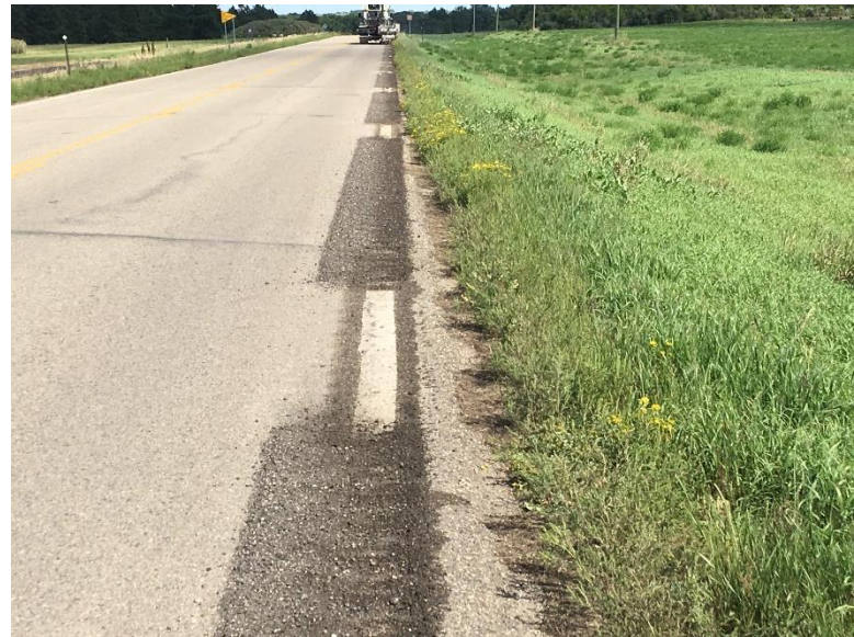
Figure 15: Rumble strips enhance Tribal transportation safety by enhancing driver alertness.
