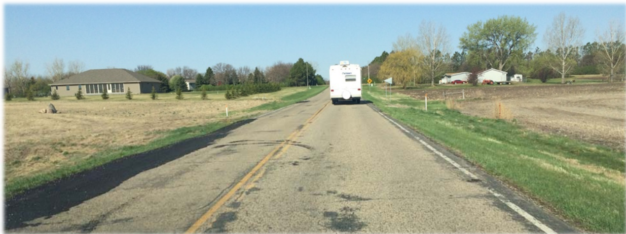
Photo of Pavement Condition of Brown County Highway 13
