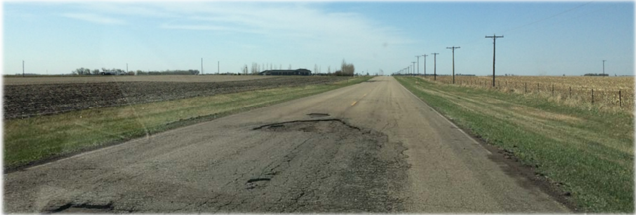
Photo of Pavement Condition of Brown County Highway 6
