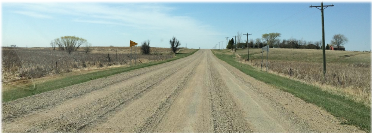
Photo of Pavement Condition of Brown County Highway 20
