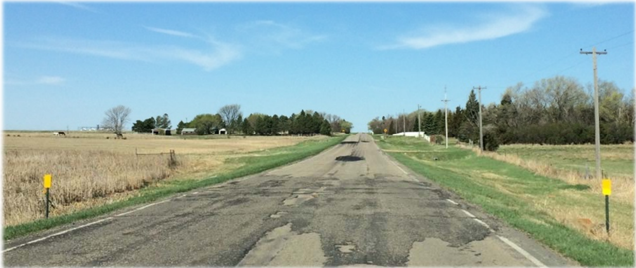
Photo of Pavement Condition on a Brown County Road
