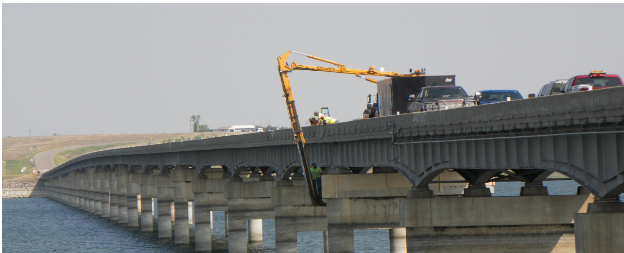
SDDOT crew members inspect the Singing Bridge for damage and work to repair and reopen it for the public.
