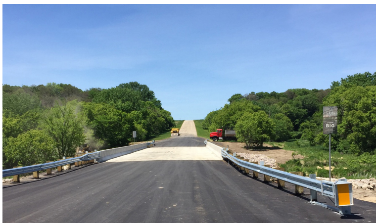
A three-span double-tee continuous concrete bridge near Sisseton was constructed over the Little Minnesota River.
