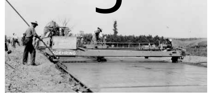
This 1939 photograph shows a Koehring longitudinal float used for portland cement concrete paving in Union County.
