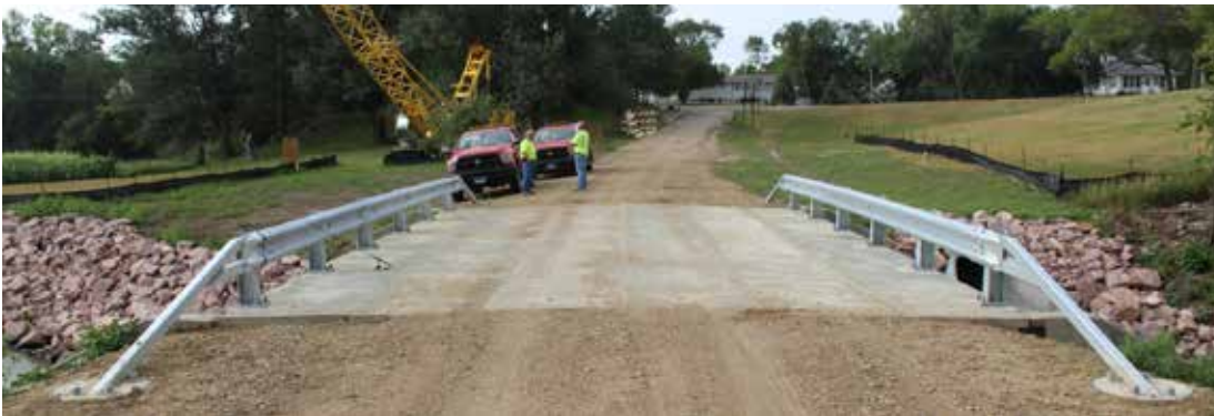
This prestressed concrete double-tee bridge on 7th Street East in Redfield, built over Turtle Creek in 2017, replaced a one-lane, guardrail-less, 25-foot steel stringer bridge with a timber deck, built in 1930. The project was paid for with federal bridge funds, plus 20 percent local matching funds.
