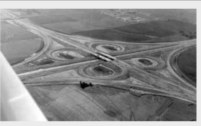
Newly graded cloverleaf interchange of Interstate highways 90 and 29 in Sioux Falls, circa 1961. Object at left is an airplane wing strut.
