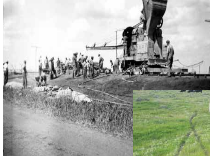
Above: This 1936 paving scene in Hand County shows how steep inslopes on early highways could be. At right: The gentle inslope on this South Dakota highway may have contributed to this driver's survival.
