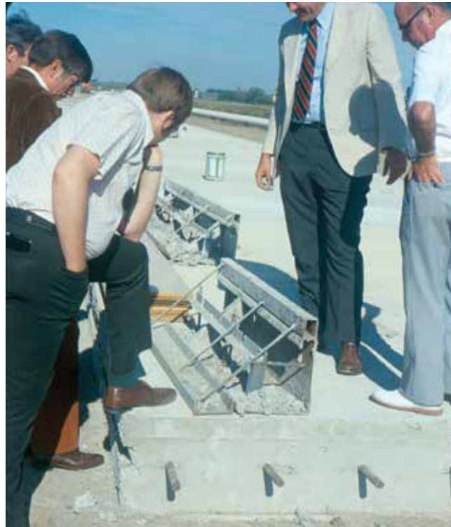
Inspection of the newly constructed east end of the east-west runway at the Sioux Falls airport in 1978
