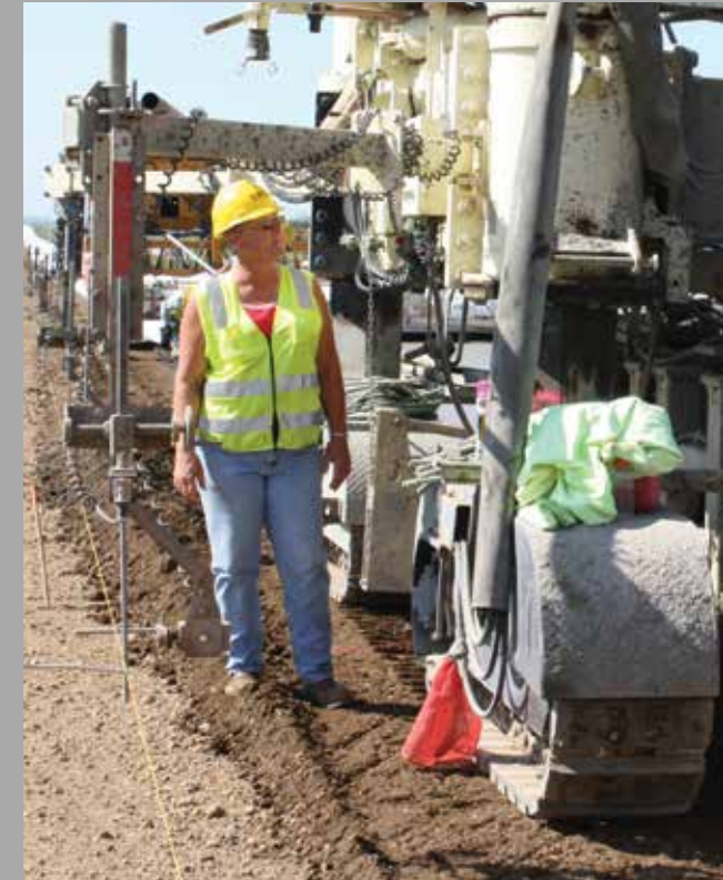
Federal stimulus funding in 2009 helped reconstruct segments of I-29 and I-90, including this northbound I-29 segment between the Beresford and Volin exits.
