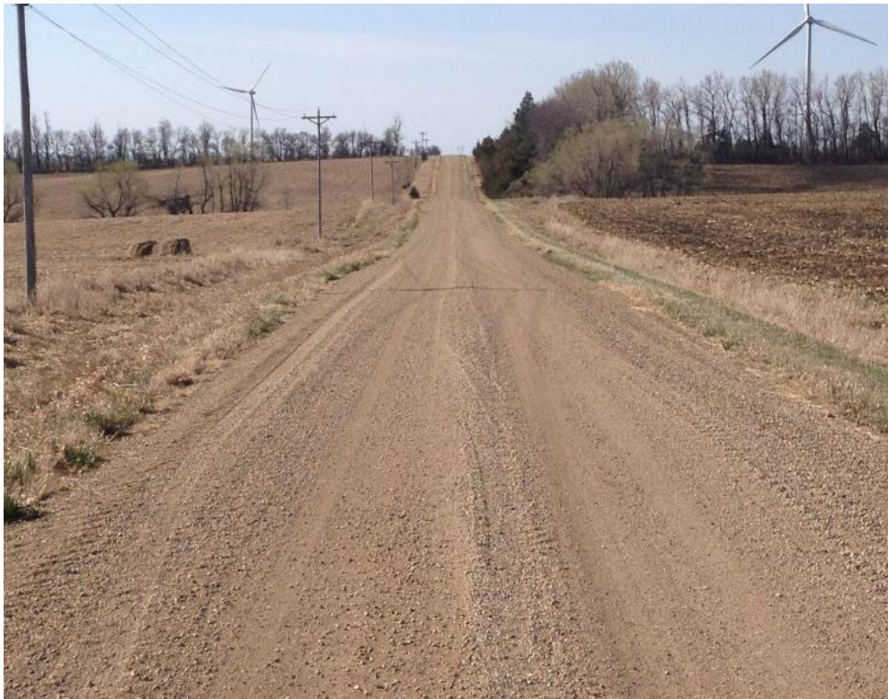
This is the same road as shown in the previous photo after complete surface and shoulder reshape and new surface gravel added. It performs well once again.
