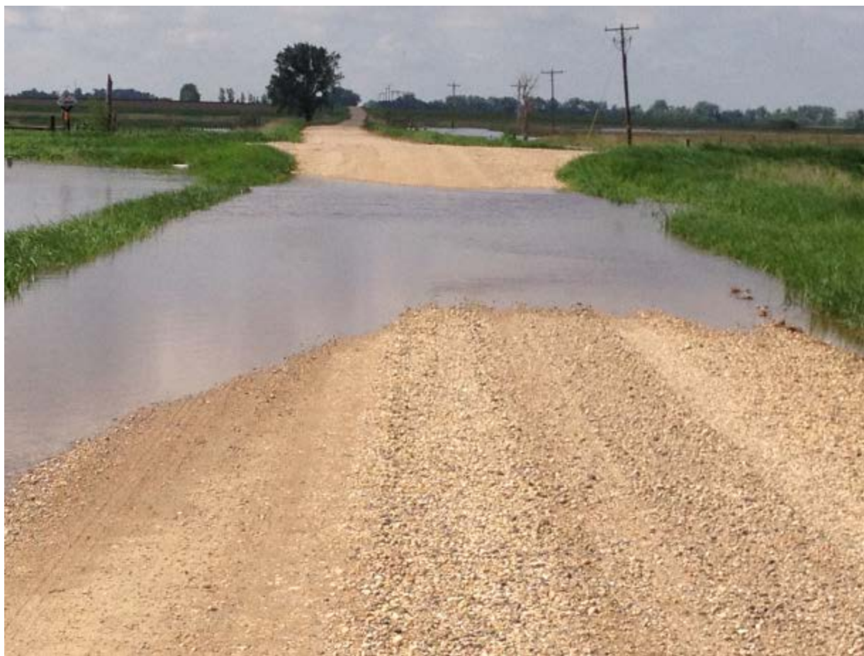
Plugged or collapsed culverts cause serious damage when water flows over roads.
