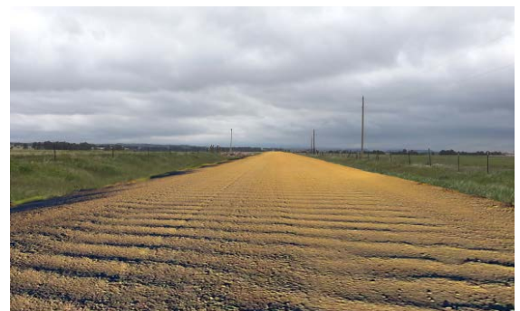
Typical washboard damage on an unpaved road (Source: Jo Michele Sheridan).
