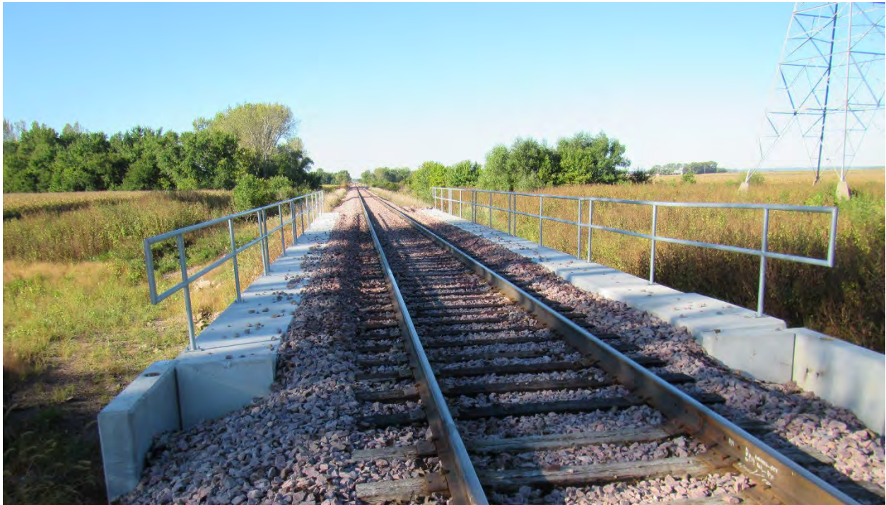
View of Bridge T-478 after replacement, showing use of pre-cast concrete tubs, ballast, and timber rail ties. The concrete walkway and galvanized railing shown here will not be applied to Bridges P-125 and P-131.
