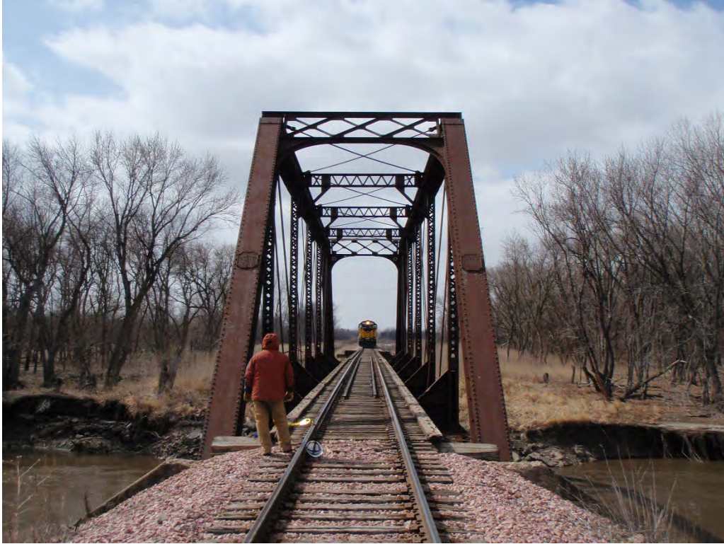
Approach view of Bridge T-480 prior to rehabilitation of the approach span.
