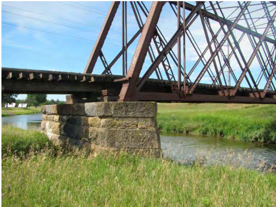
Figure 26. View of deteriorating support column, Bridge P131, facing southwest.
