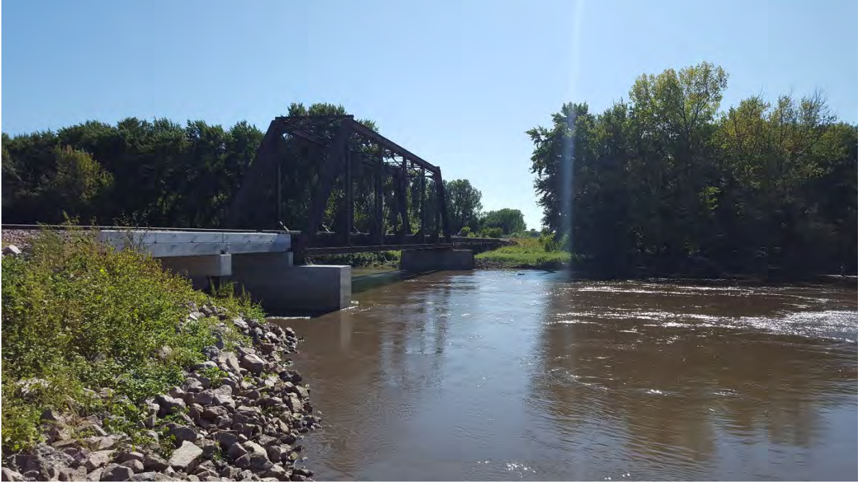
Quarter view of Bridge T-480, showing use of replacement materials at the approach span.
