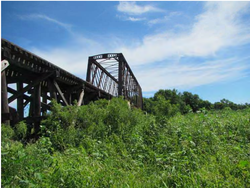
Figure 10. Overview of the trestle approach and truss structures, Bridge P106, facing east-northeast.
