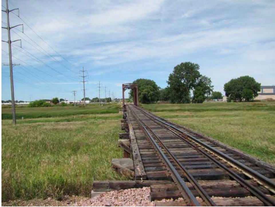
Figure 21. Overview of timber trestle and steel truss structures, Bridge P131, and site 39MH2014, facing west.
