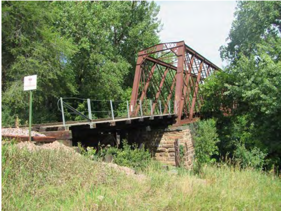
Figure 16. View of south timber trestle approach and steel lattice through truss structures, Bridge P125, facing north-northwest.
