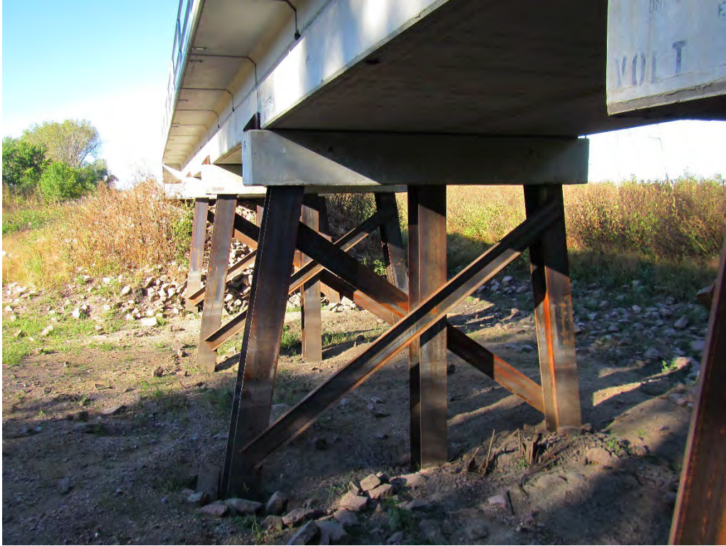
View of the steel bent substructure at Bridge T-478. The steel was installed to replace the timber trestle that had reached the end of its service life.
