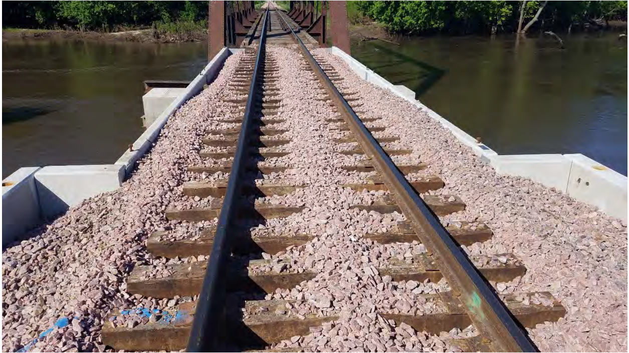
Approach view of Bridge T-480 showing the use of pre-cast concrete tubs. The scope of the rehabilitation of Bridge T-480 is greater than the proposed work at Bridges P-125 and P-131. The masonry piers supporting Bridges P-125 and P-131 will remain.
