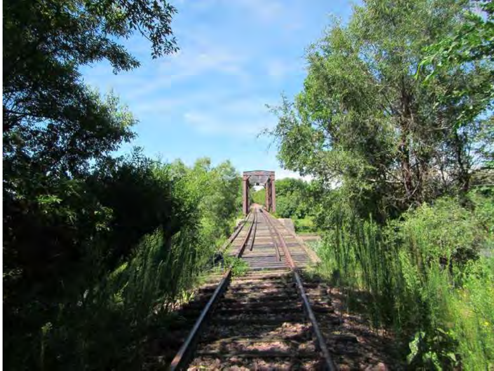
Figure 13. View of east trestle approach and truss structures, Bridge P106 and site 39MH2003, facing west.
