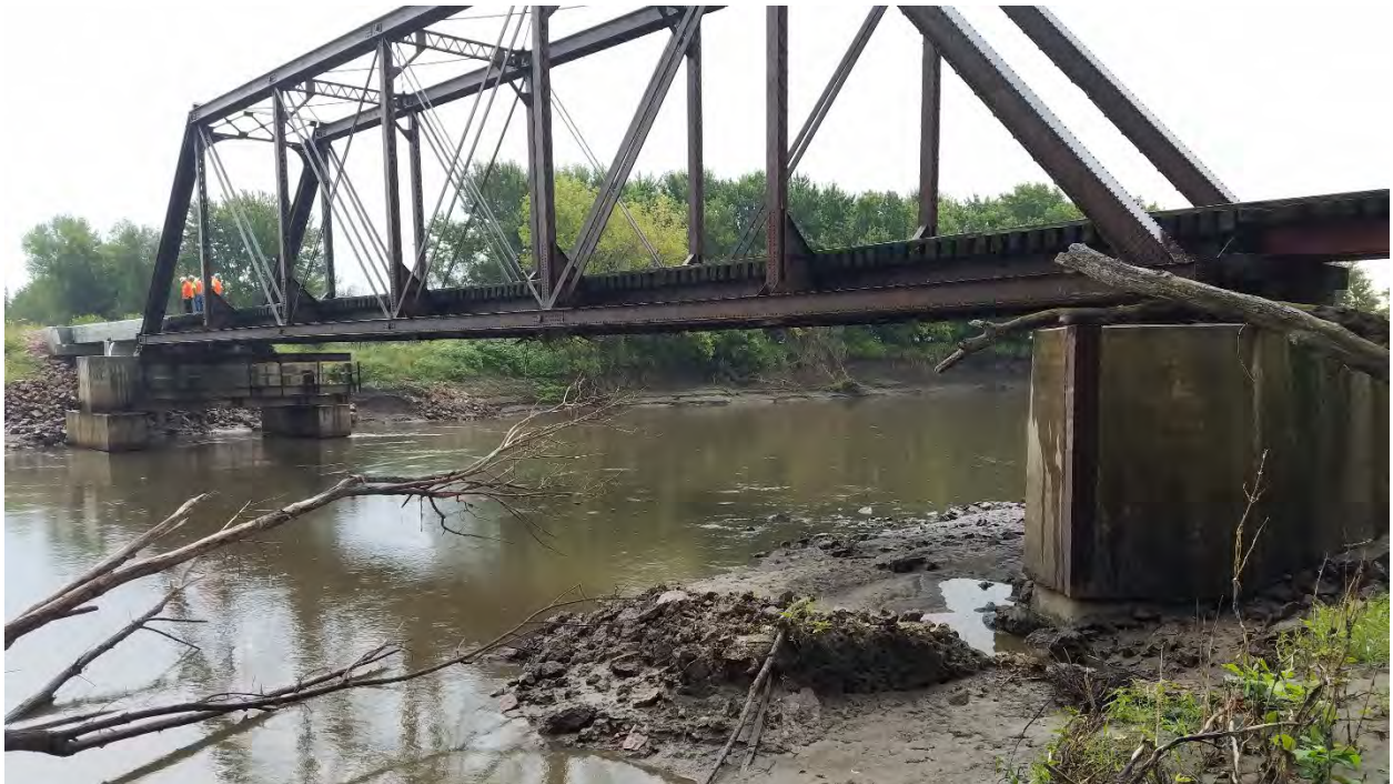
Profile view of Bridge T-480 showing the use of replacement materials, at left.
