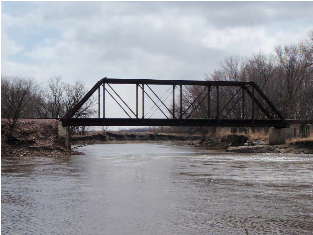
Profile view of Bridge T-480 prior to rehabilitation of the approach span.
